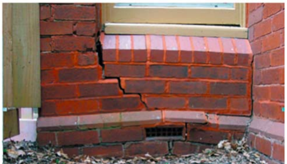
(Typical building foundation damage due to differential soil movement)
